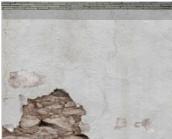
04. Damaged Render Wall - 1.8m
