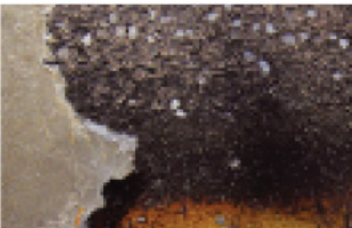
14. Burnt / Damaged Metal
